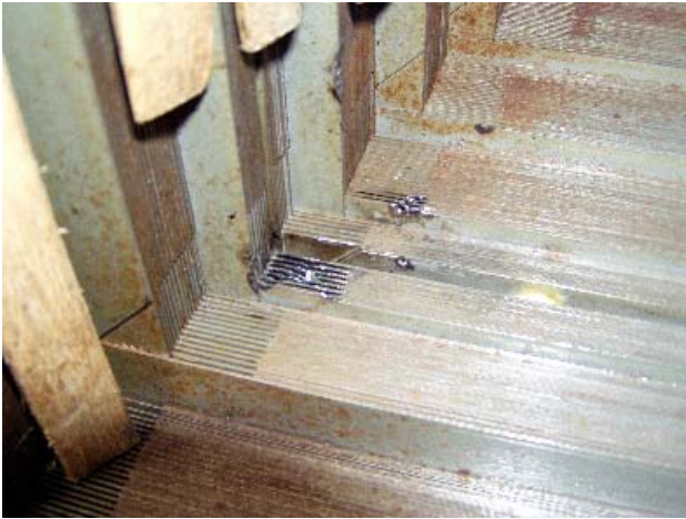
Fig.1 The fault of the 220kV power transformer was found after returned to factory
