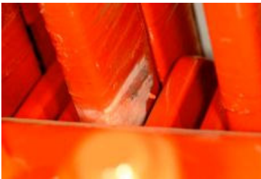
Fig.15: Severe degradation due to spark discharges caused by ageing of the semi-conducting coating at an endwinding
