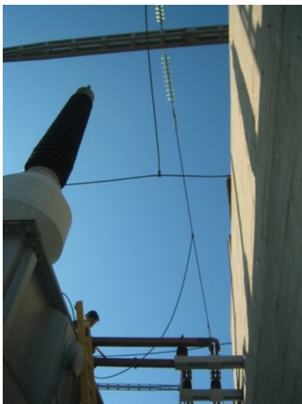
Figure 7 :230 kV line close to the transformer
