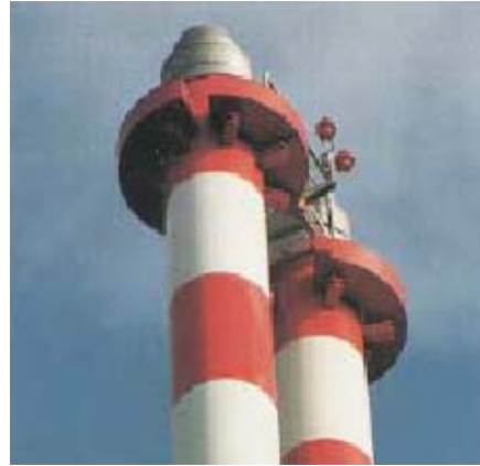
Figure 1. Tuned Liquid Dampers (TLDs) installed in chimneys.
