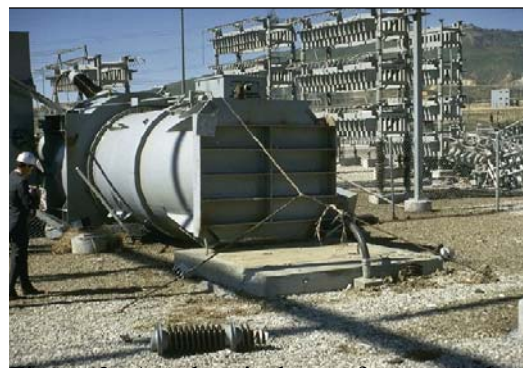
Figure 2. An electrical transformer at the Sylmar Converter Station, California, that overturned during the 1971 San Fernando earthquake.
