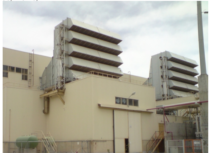
Figure 2: Khoramshahr power plant V94.2.5 Gas Turbine air intake units
