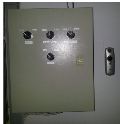
Fig. 4. Central control panel (left) and shading system remote control (right)
