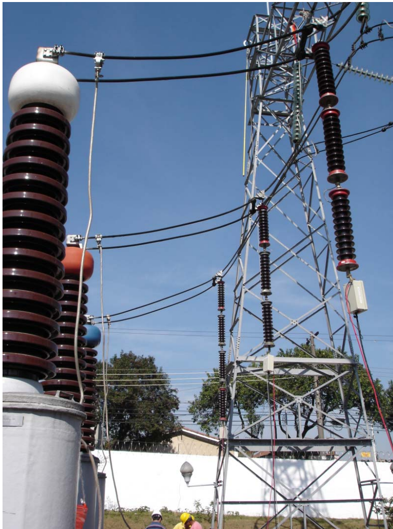
Fig. 22 Setup for the measurement of the residual voltage of an underground transmission line (length 9km, voltage 230kV) after disconnection from power source. Capacitive dividers are shown at the right side.
