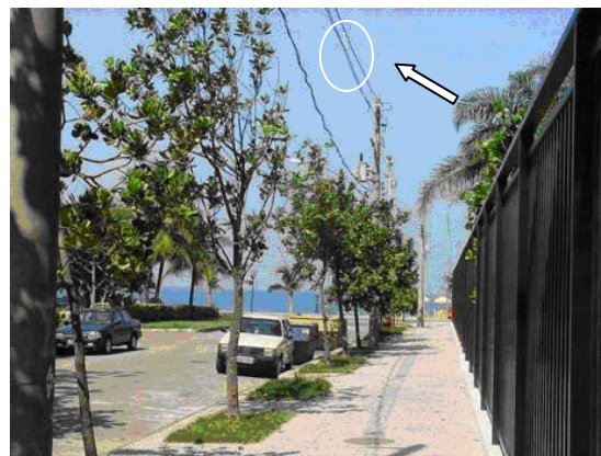
Fig.3 – Distribution line near the coast.
