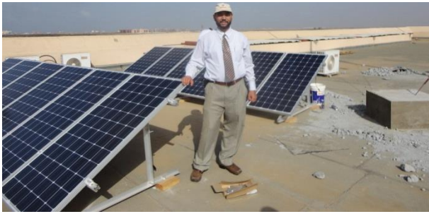
Figure 18, Installed PV Array [18]
