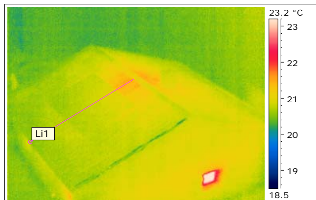
Figure 14: Roof infrared imaging (after 20min without double internal insulation)
